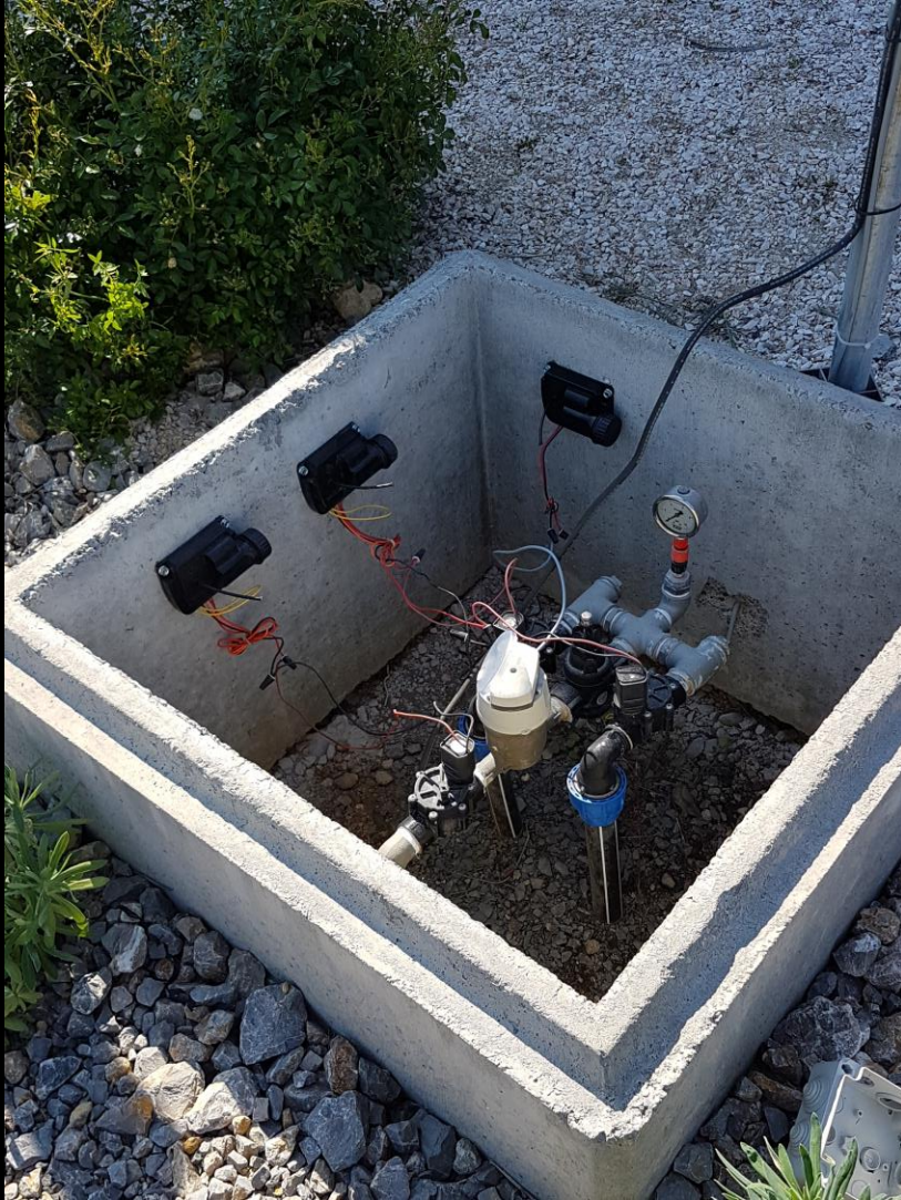
concrete valve box
